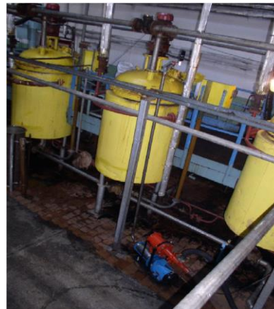
Fig. 1. Cavitation bifrequency installation in the production line at the Chisinau canning factory
