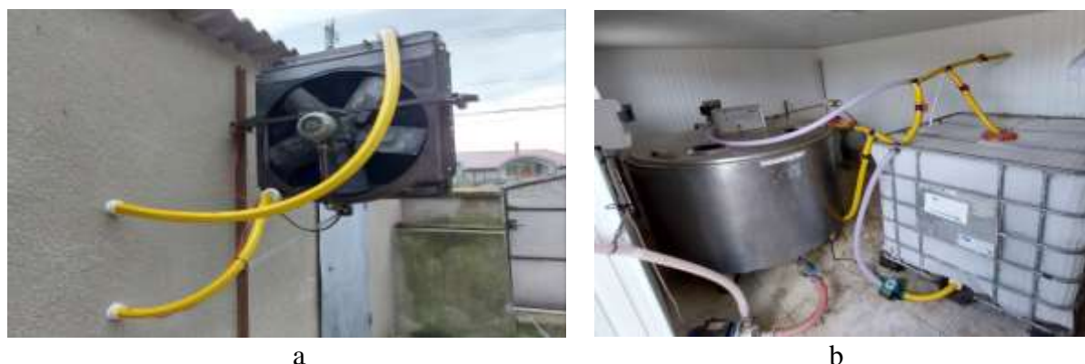
Fig. 11 Experimental refrigeration plant, combined with artificial and natural cold a – section of the refrigeration plant outside the PCL b- section of the refrigeration plant inside the PCL
