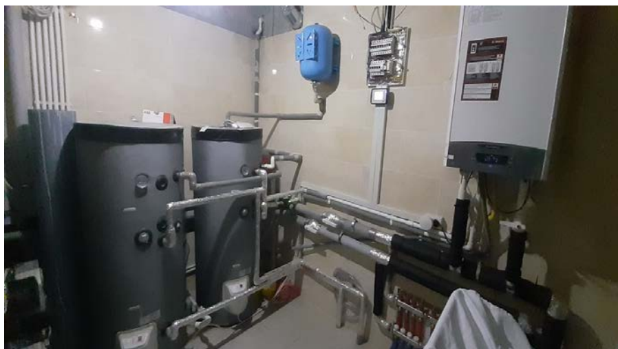
Figure 5. Gas boiler and hot water boilers.
