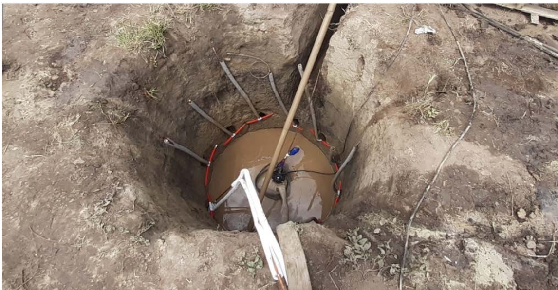
Figure 2. Geothermal circuit of the heat pump in the village of Cania. (SRL "Climatehnic" photo)
