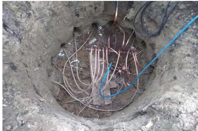
Figure 4. Geothermal circuit of the heat pump in the city of Comrat. (SRL "Climatehnic" photo)
