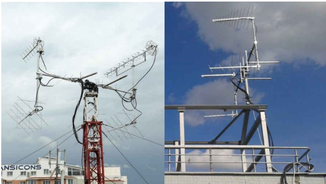
Figure 5.1. Views of ground stations developed at NCST TUM.
