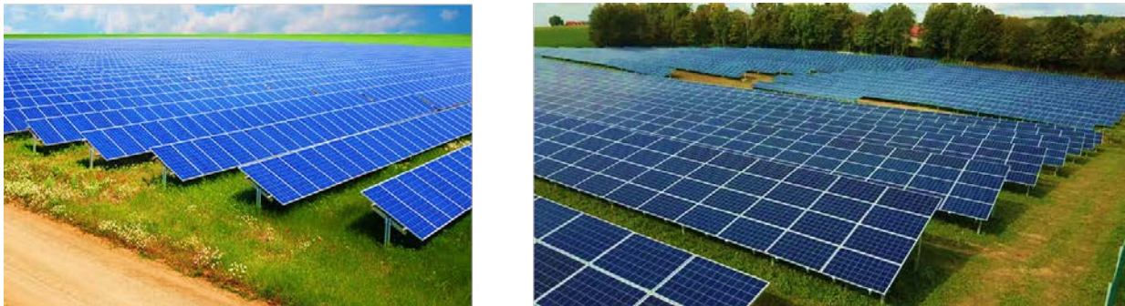
Figure 4. Real PV implementation of design V1 (left) and V2 (right) geometry.
