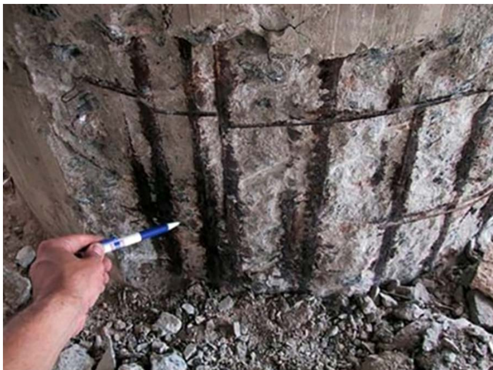
Figure 1. Chemical corrosion of cement stone.
