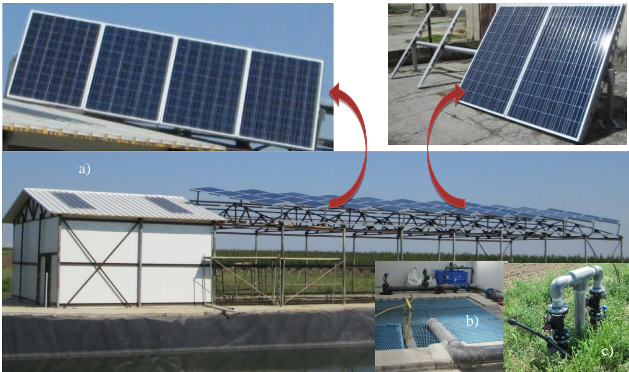
Fig. 12. Components of the photovoltaic plant with installed power P = 11 kW: (a) - Mounting of PV panels in housings with ability of rotating around the central axis; (b) – the pumping station hall; (c) – the central water supply pipeline of the irrigation system.
